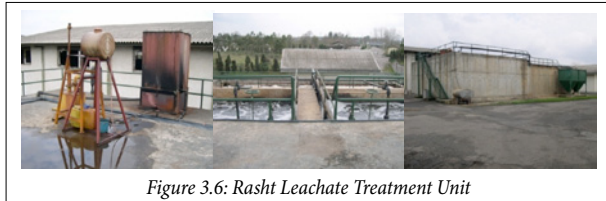
Figure 3.6: Rasht Leachate Treatment Unit
