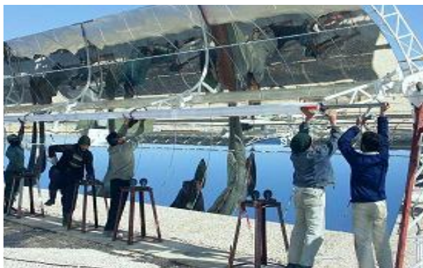
Shiraz Photovoltaic Project, Fars Province
