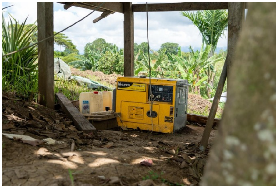
Figure 23. The diesel generator used at the case study farm
