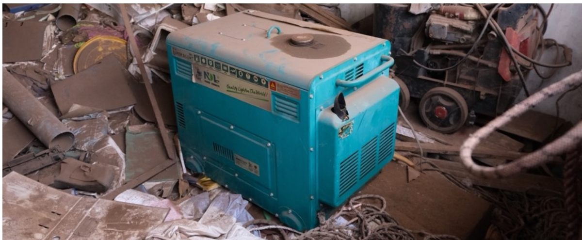
Figure 20. Diesel generator at the Abuko market and slaughterhouse (June 2024)
