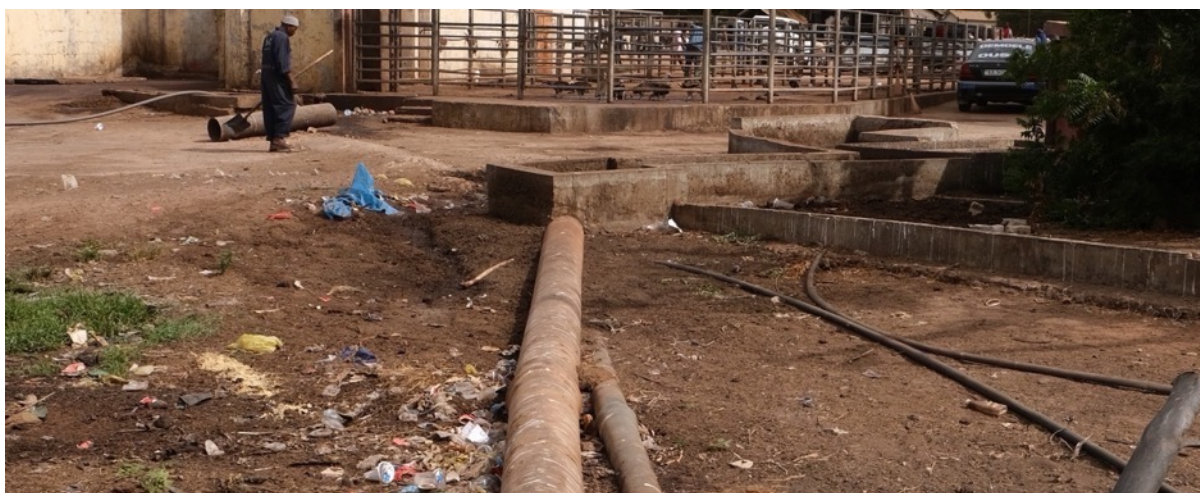
Figure 19. Slaughterhouse wastewater SWW system (June 2024)
