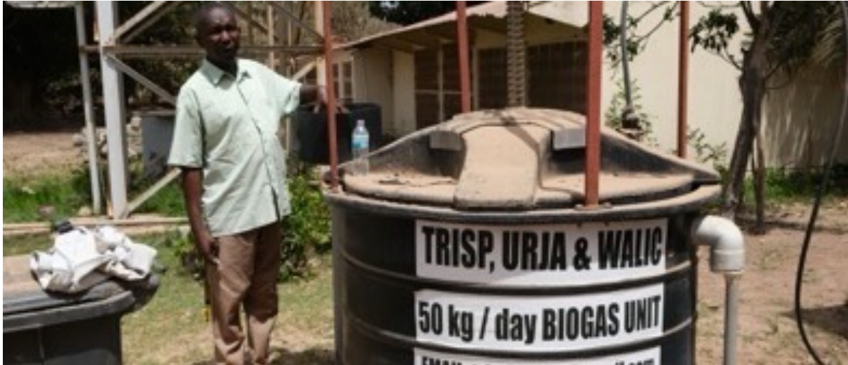
Figure 2. First-ever biogas plant in The Gambia (June 2024)
