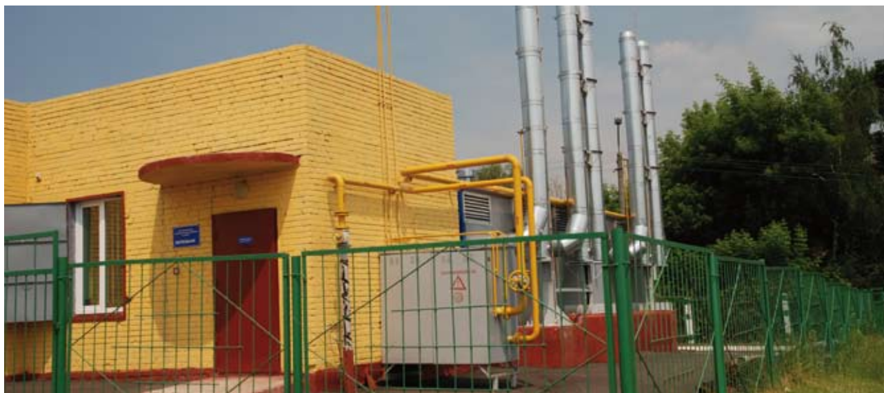
UNDP-GEF Project, “Removing Barriers to Greenhouse Gas Emissions Mitigation through Energy Efficiency in the District Heating System in Ukraine”. Module type individual boiler plant constructed for Humanitarian Gymnasium Complex and Swimming pool in the city of Rivne, Ukraine, in 2008, allowed avoiding significant heat losses at utility’s 2km manifolds and secured first comfort winter for schoolchildren and teachers since 1994.
