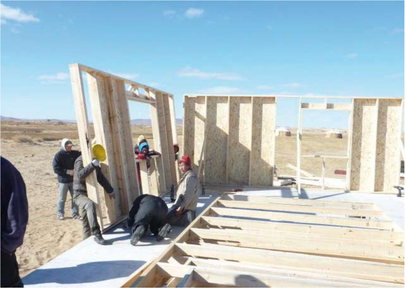
Energy Efficiency Buildings in Mongolia: Wall erection for a timber-frame house © Ts.Battur
