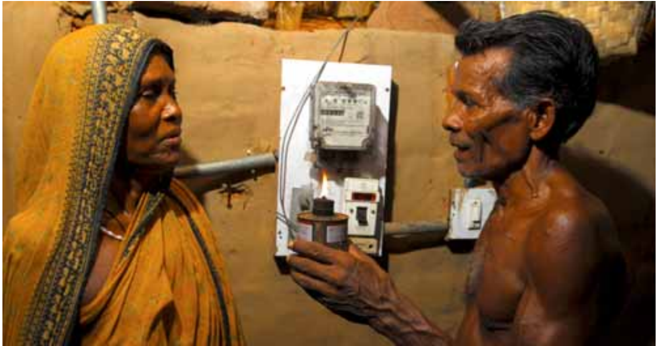
Electricity access to poor houses. Project: Rajiv Gandhi Grameen Vidyutikaran Yojana (RGGVY) – India
