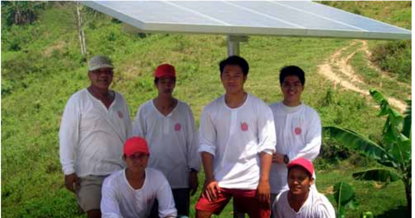
Erecting a solar photovoltaic system. Project: Accelerating Community Electricity Services using Solar (ACCESS) – the Philippines.
