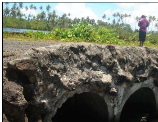
Box culverts help water flow more easily during severe flooding
