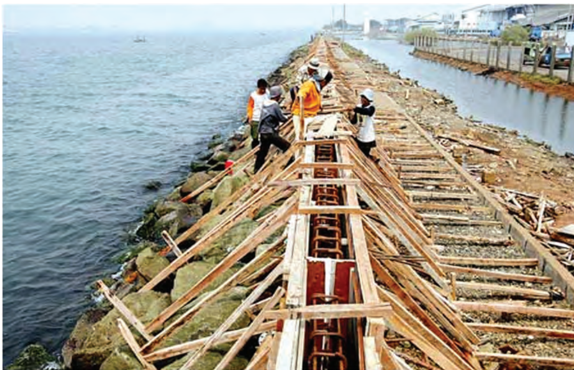
Figure 4.38 Construction of a dike to reduce flooding from high tides and extreme waves in East Harbour of Muara Bary, Jakarta. Source: Media Indonesia, 2007
