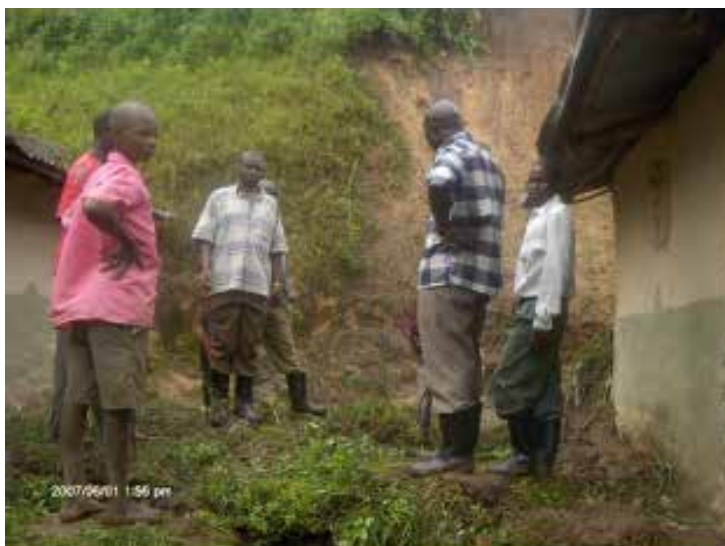
Figure 1: A landslide could result from hill crosscutting for house construction due to rapid population growth in the upstream communities (Source: NEMA, 2010)
