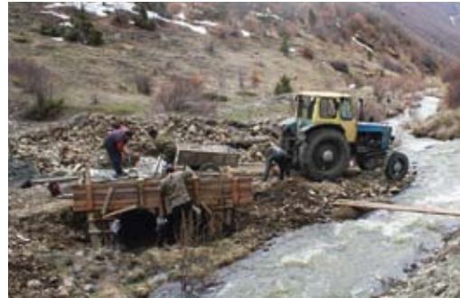
Rehabilitating field roads in Tsapatagh facilitates better access to summer pastures and helps fight erosion & overgrazing in winter pastures
