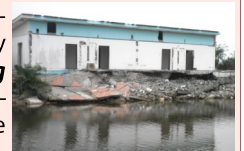
A home destroyed from erosion in Montserrado County
