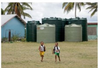
The Lofeagai community installed a water cistern: the first storage capacity for this community. Now, 90% of the Lofeagai population has access to the necessary minimum water supply of 40 liters per day, even during periods of extreme drought. Photo: Joe Hitchcock & Luke McPake
